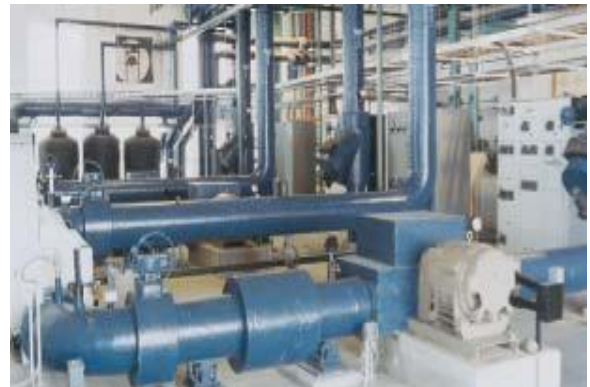
FOAMGLAS® insulated chilled water piping
