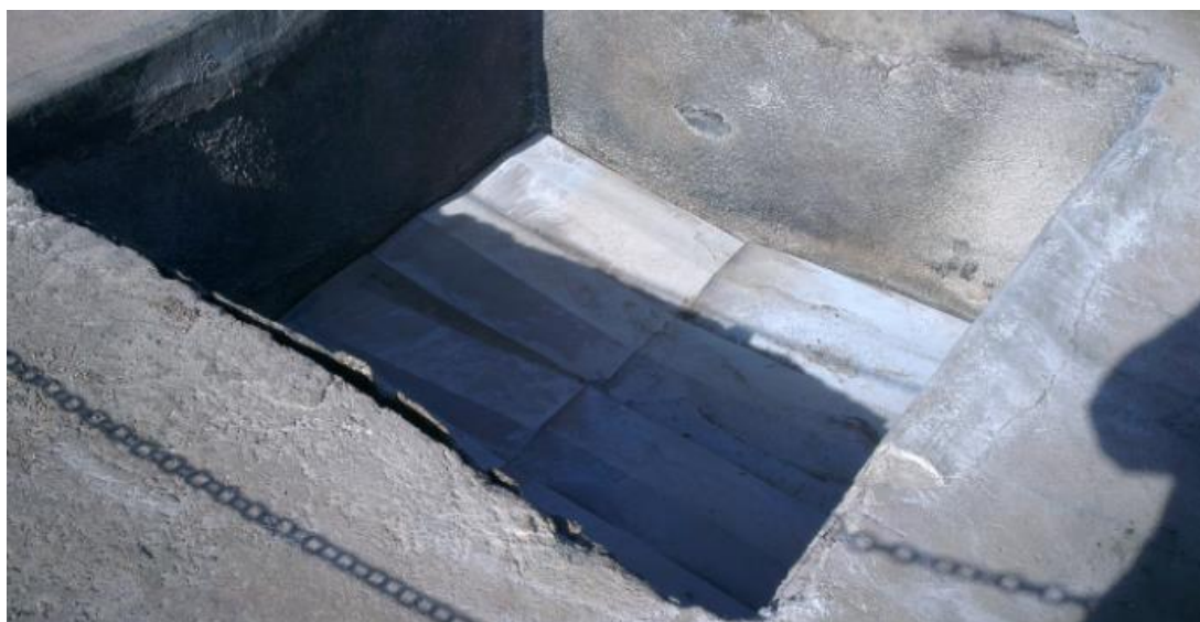
Figure 19: FOAMGLAS® PFS System (Gen 2), after the fire was extinguished using dry chemical
