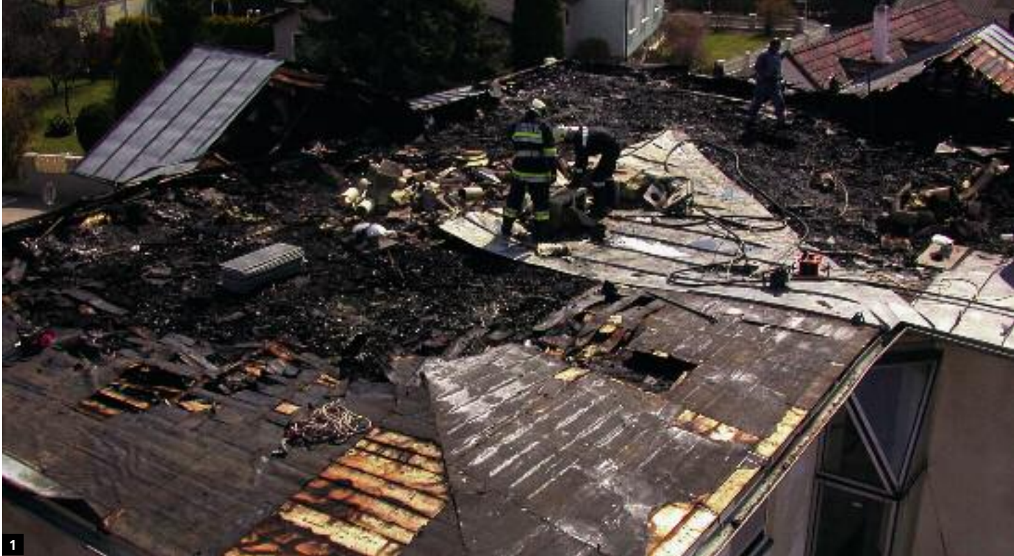
1 The propagation of fire across the roof can cause total damage on the building.
