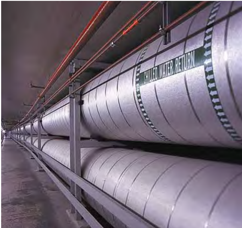
Chilled water piping at NIH.
