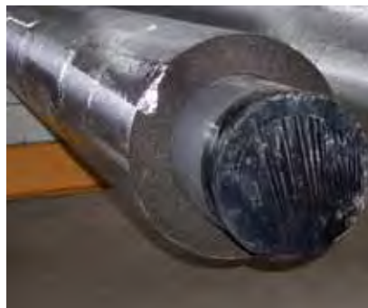
Chilled water piping at Dublin International Airport.
