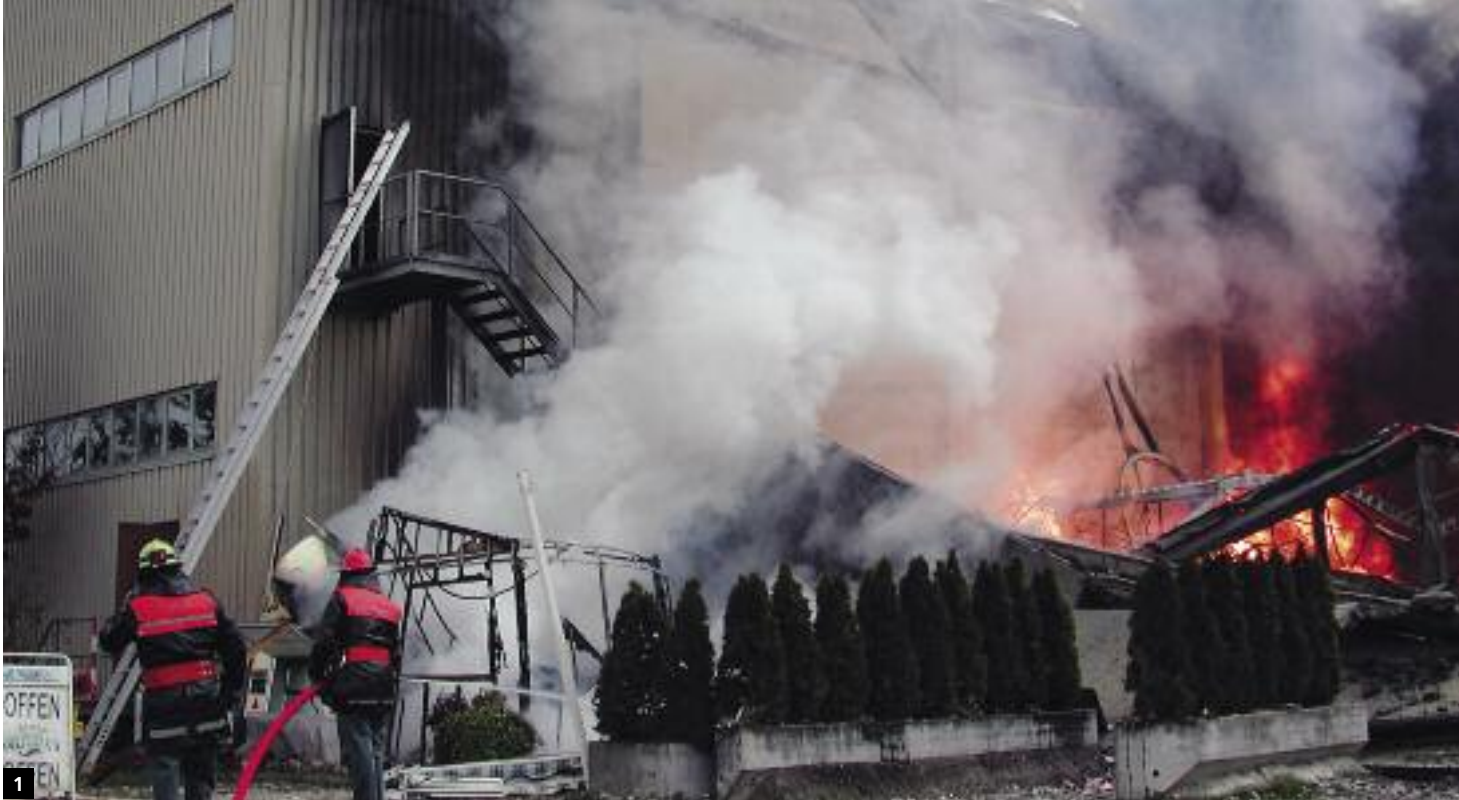
1 The spread of fire across the façade and the roof can contribute to devastating total loss.
