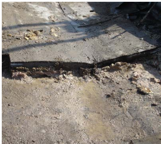
Amount of condensed moisture within the roof build-up can be enormous
