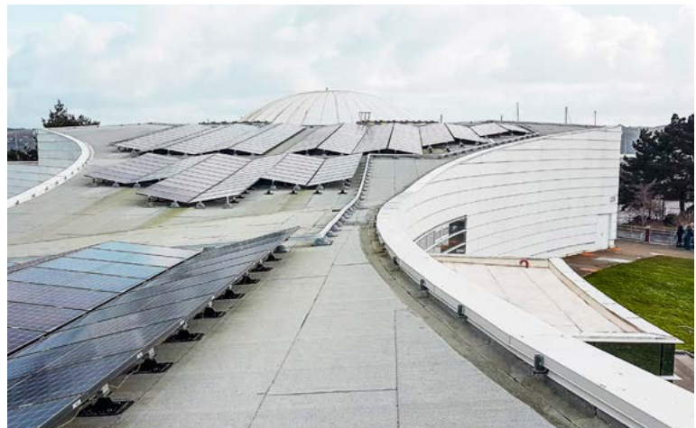
Photovoltaic roofs Océanopolis, Brest, France
