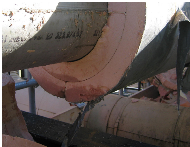
Moisture accumulation in PU foam system due to breach in vapor barrier.
